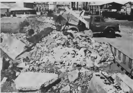
THE NORTH side of Lago's original reservoir has been pushed over giving access to trackloads of debris which will be used to fill and level the cavity that once held 4392 barrels of water.
